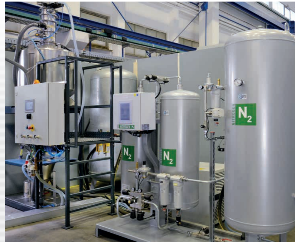
Nitrogen generator The nitrogen generator permits the creation of the inert gas atmosphere with a nitrogen purity of up to 99.9%.
