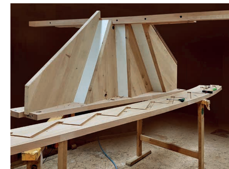
The unit is used to capacity and Ammann produce components for 30-35 stairs a week.
